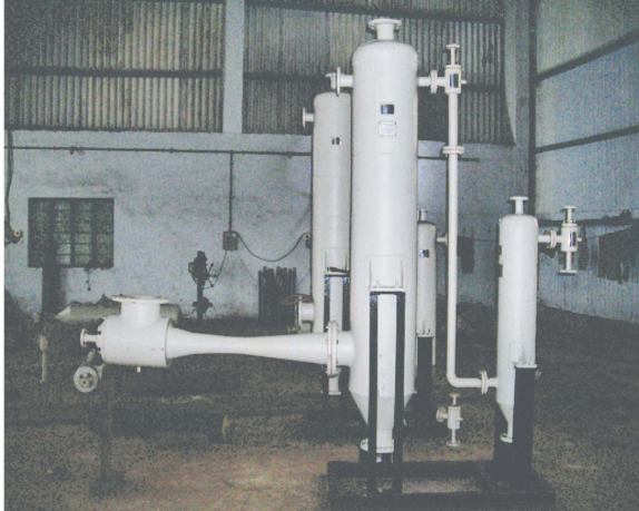
Double Stage Vacuum Booster (edible oil refinery)
