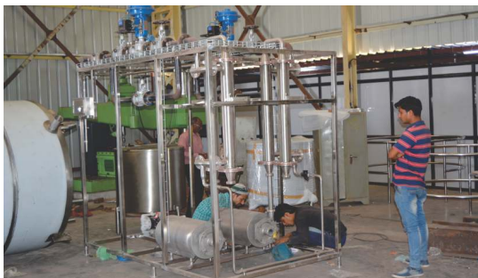
CIP High Pressure Water Distribution Skid
